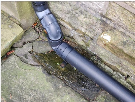
Photo - 11 Leaking downpipe at front door
