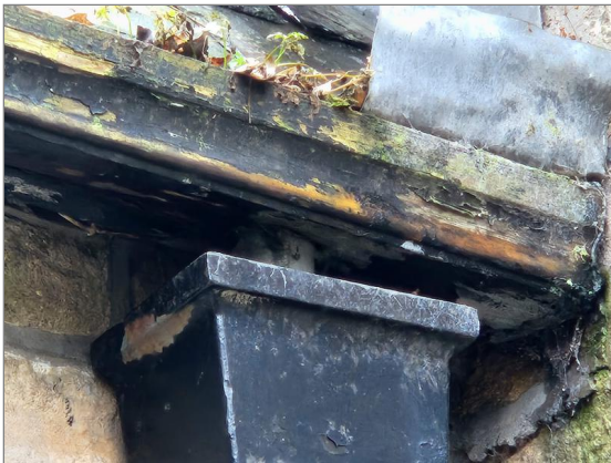
Photo - 9 Repair/replace timber gutter at rear
