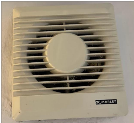
Photo - 28 Bathroom extractor.
