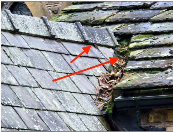
Photo - 7 Slates ok - localised pointing plus blocked rear valley gutter
