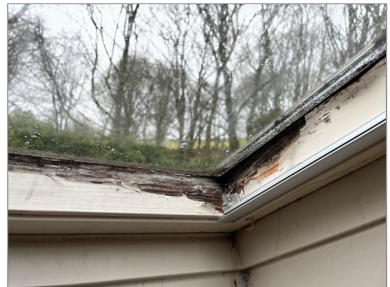
Photo - 15 Rear bedroom Velux rooflight - neglected.
