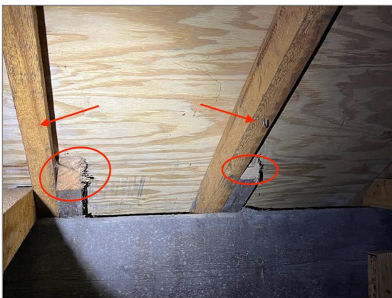
Photo - 20 Replacement rafters (arrowed) and originals cut short (circled).
