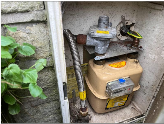
Photo - 32 Gas meter.
