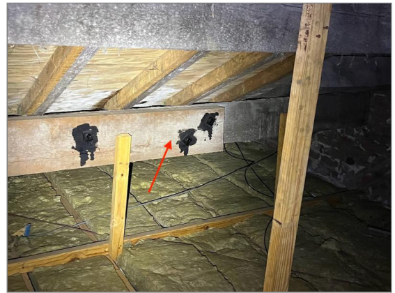
Photo - 17 Roof structure - replacement purlin arrowed.
