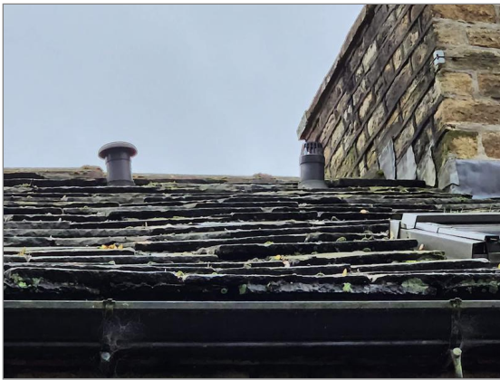
Photo - 1 Soil vent pipe and bathroom extractor which pass through the rear roof slope.
