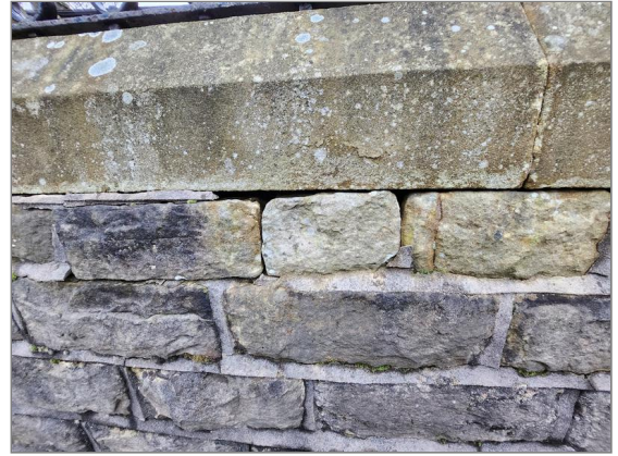
Photo - 39 Localised pointing to front retaining wall
