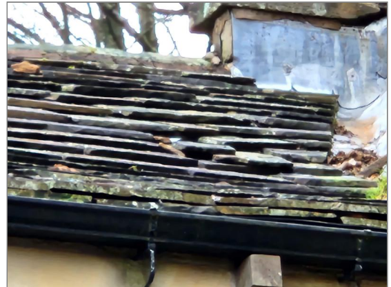
Photo - 4 Slipped slates / loose pointing
