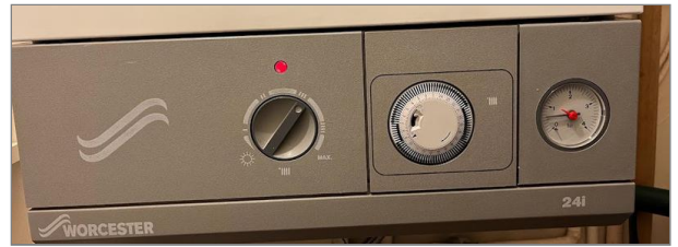
Photo - 35 Boiler control panel and model detail.
