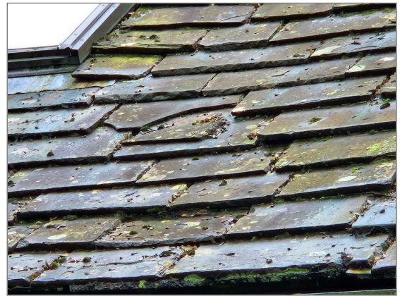
Photo - 8 Cracked slates at rear
