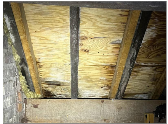
Photo - 2 Damp secondary water proof layer (sarking board).
