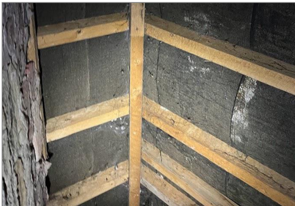
Photo - 24 Rear addition / utility roof structure and secondary waterproof layer (roofing felt).
