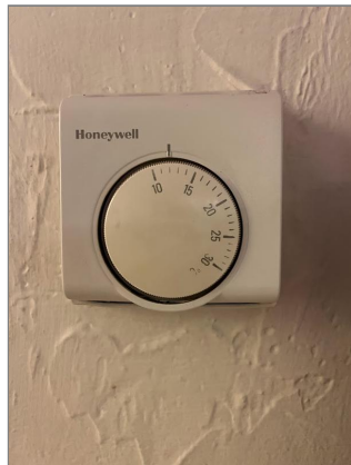
Photo - 36 Room thermostat.
