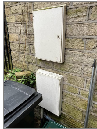
Photo - 33 External meter boxes.
