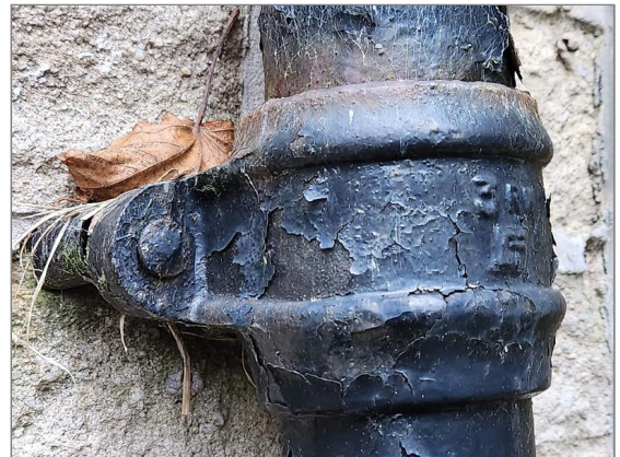
Photo - 10 Rusted rear downpipe
