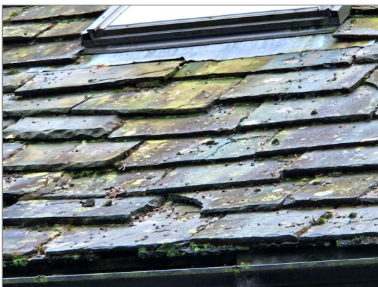
Photo - 5 Cracked slates on rear slope
