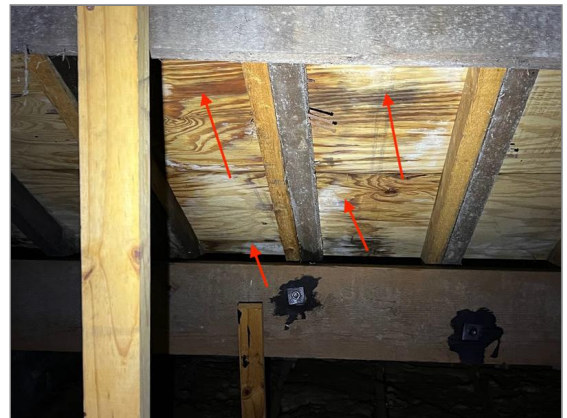
Photo - 19 Damp penetration.
