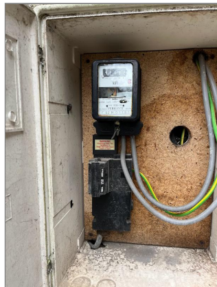
Photo - 31 Electricity meter and incoming supply.
