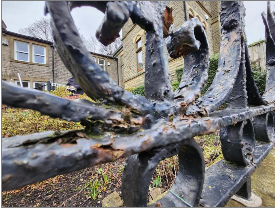
Photo - 38 Railings rusted at front
