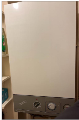
Photo - 34 Central heating boiler.
