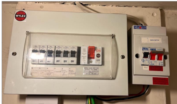
Photo - 29 Dated consumer unit - no RCD protection.
