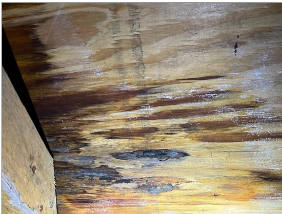
Photo - 18 Damp penetration.
