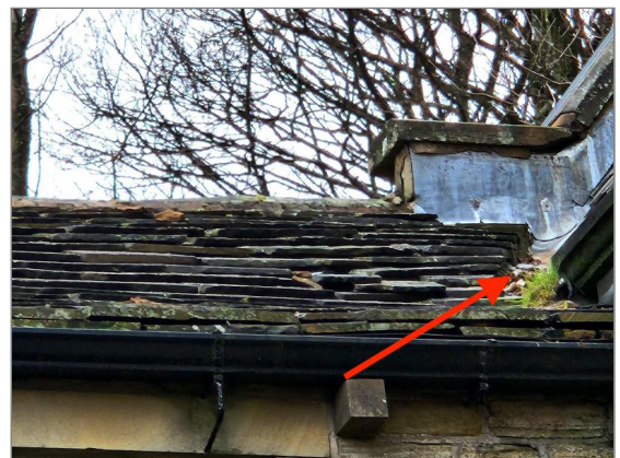
Photo - 6 Blocked valley gutter front
